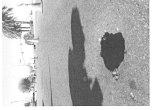
Mission Blvd Sinkhole - Before
