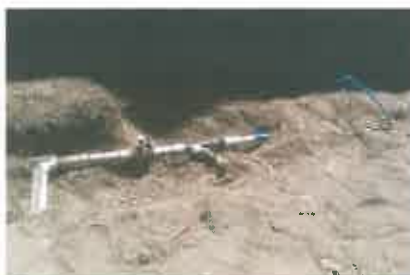
Brand new valves, pressure regulators and filters connecting to the new HDPE irrigation lines.
