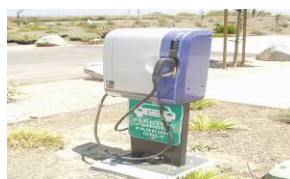
Electric Vehicle Charging Station
