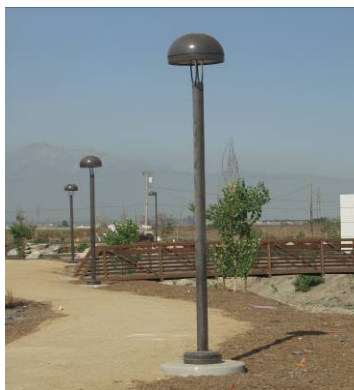
Outdoor Light Fixtures
