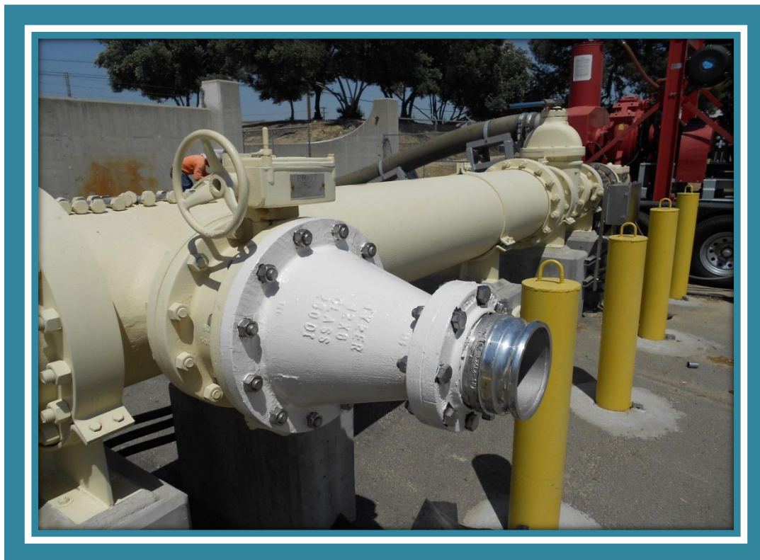
PHILADELPHIA PUMP STATION EMERGENCY BYPASS SYSTEM
