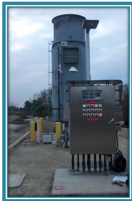
REGIONAL WATER RECYCLING FACILITY NO. 2 - FLARE & CONTROL PANEL
