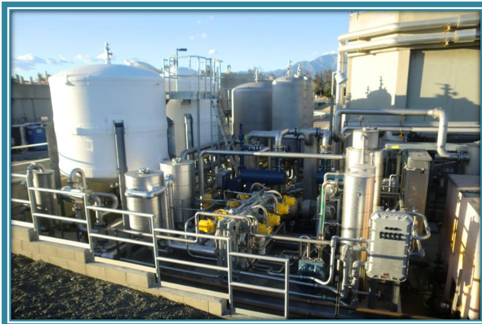
REGIONAL WATER RECYCLING FACILITY NO. 1 - FUEL CELL
