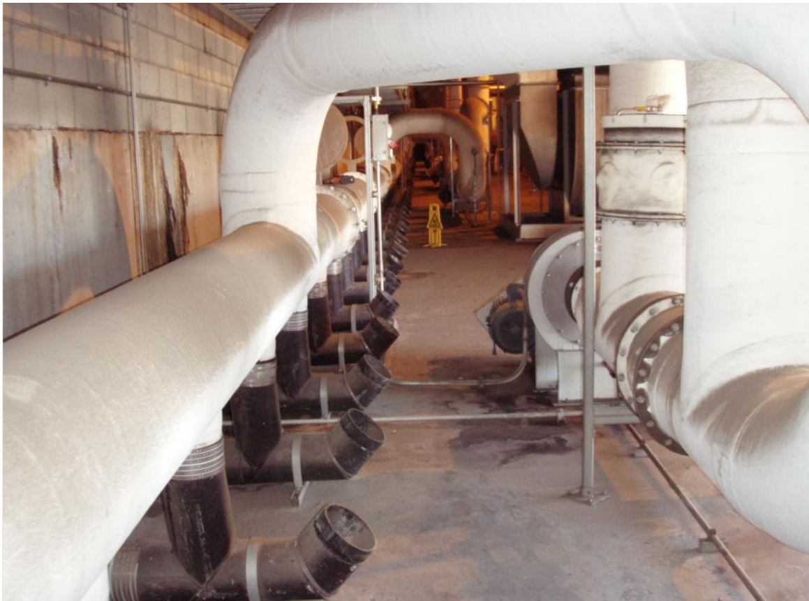
IERCF Ventilation Cleaning
