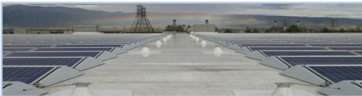
Solar panels at the Inland Empire Regional Composting Facility (IERCA)
