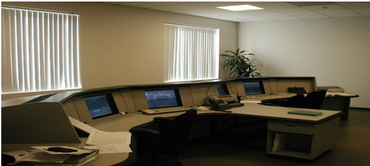
Regional Plant No. 5 - Control Room
