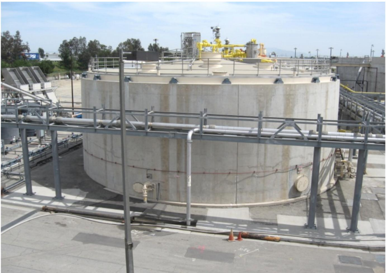
Digester No. 3 - Regional Plant No. 1 – Ontario, CA
