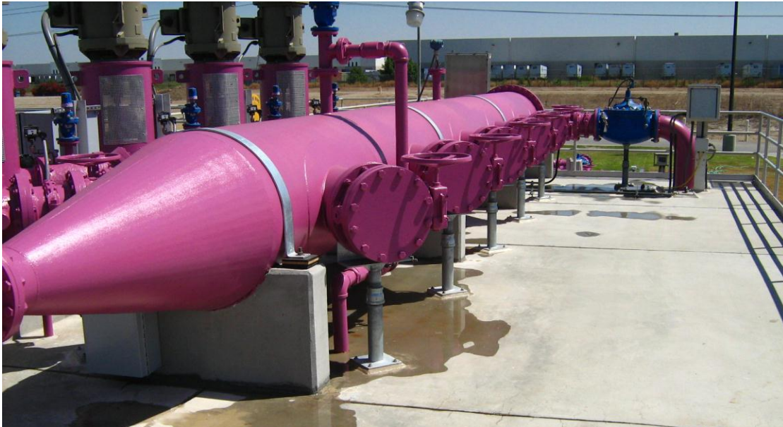
Regional Plant No. 5 Recycled Water Pump Station
