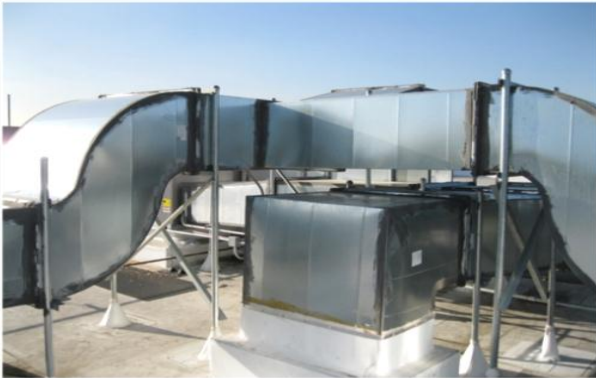
Headquarters AC System – Chino, CA
