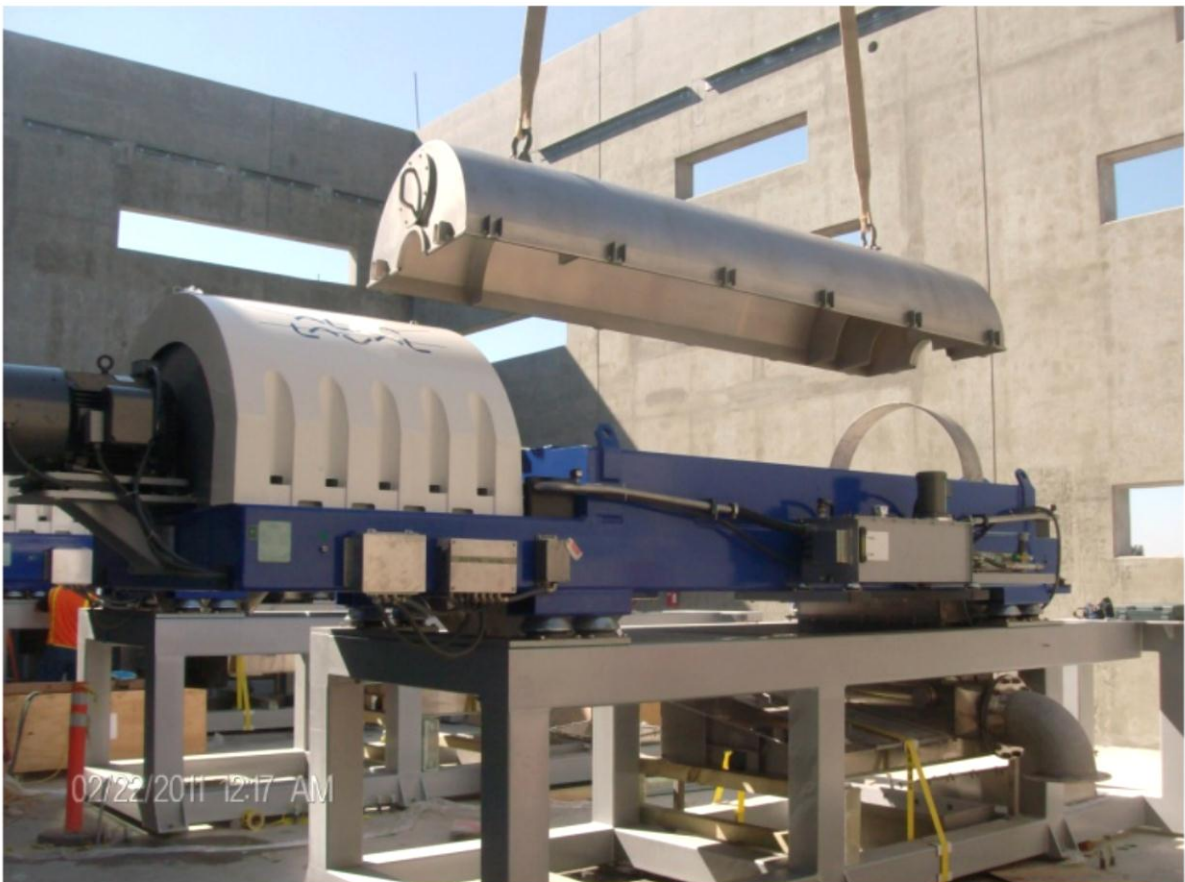
Dewatering Centrifuge – Regional Plant No. 1 – Ontario, CA
