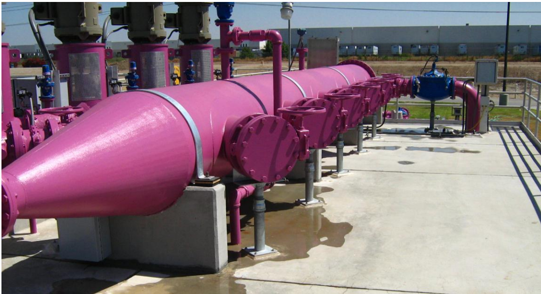
Regional Plant No. 5 Recycled Water Pump Station
