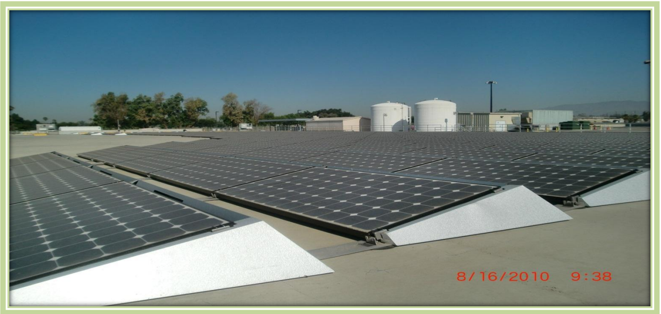
Regional Plant No. 1 Solar Panels - Ontario, CA
