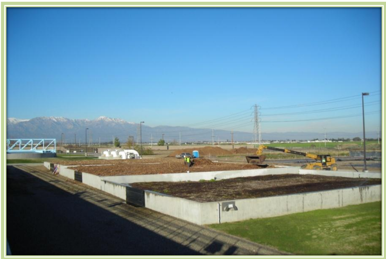
Biofilter Media Replacement
