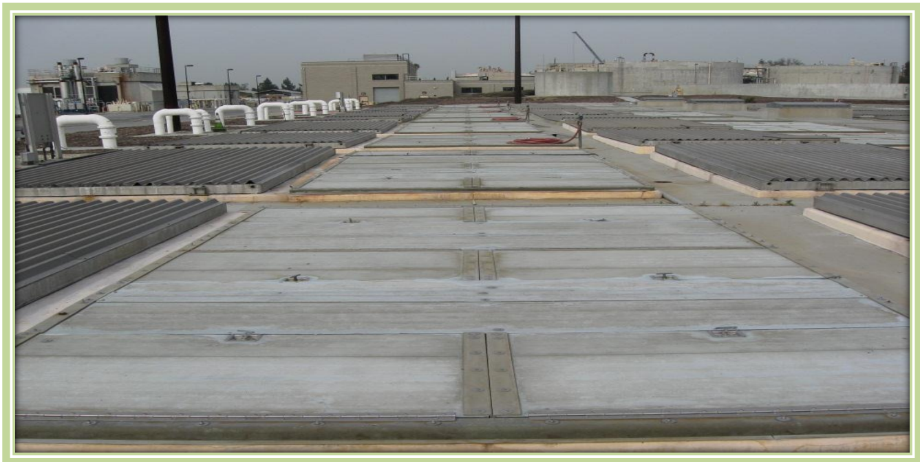
Top of Primary Clarifiers RP-1 – Ontario, CA
