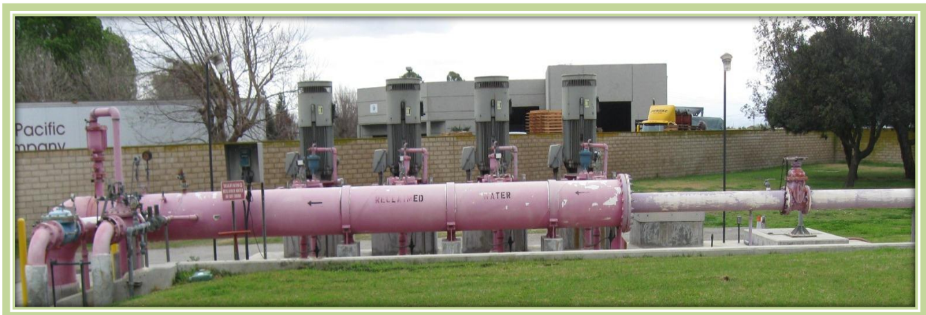
CCWRF Recycled Water Pump Station – Chino, CA
