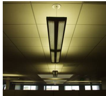
Interior Light Fixtures
