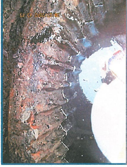
Clarifier drive main gear condition
