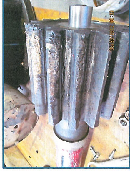
Clarifier drive pinion gear condition
