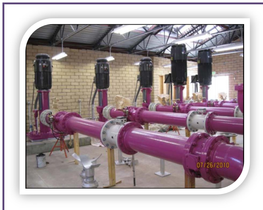
Regional Plant No. 5 Pump Station
