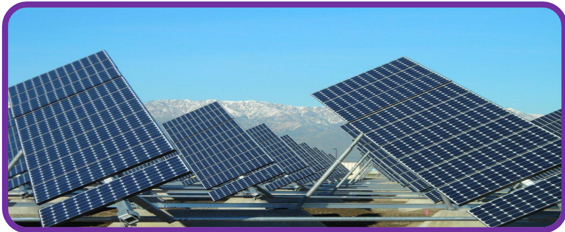
IEUA Solar Field
