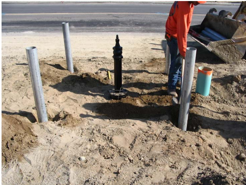
Blow-off for Pump to Waste Line
