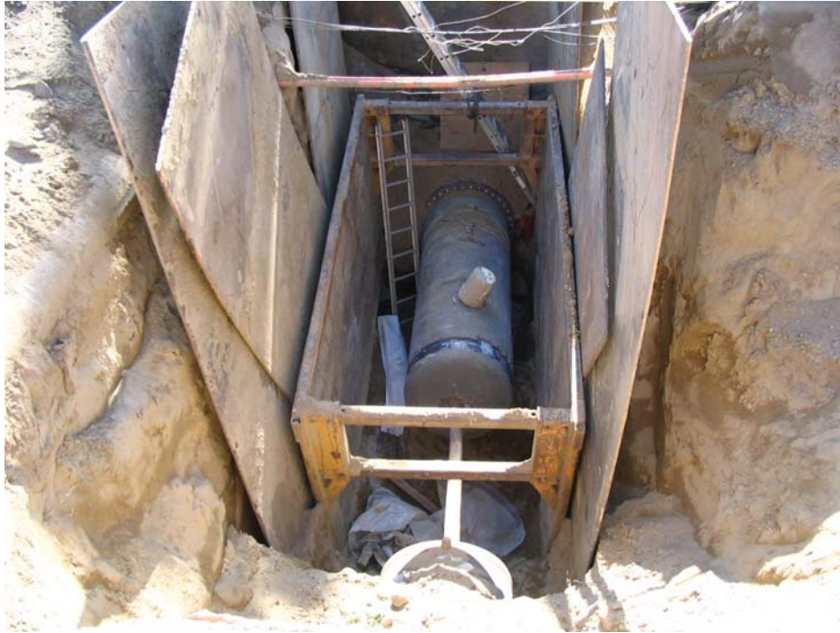
Connection to Ontario Pump Station
