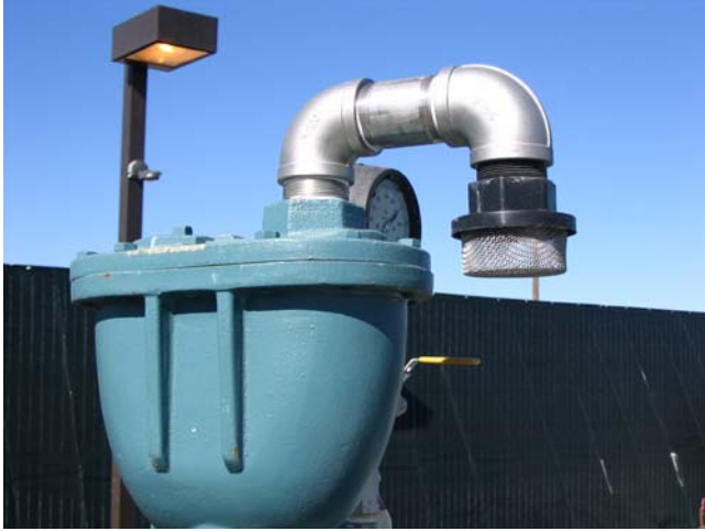
Well II-2 Screens on Air Vacuum and Air Release Valve
