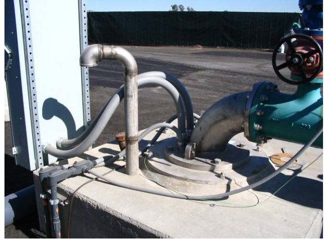
Well II-2 Air Vent Turn-Down Pipe
