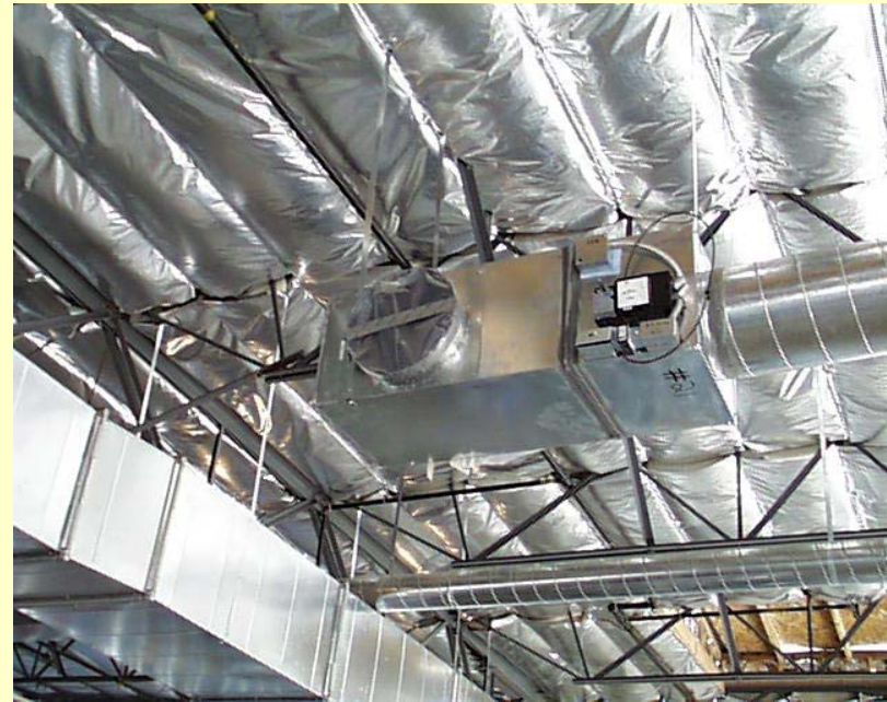
Covered HVAC ducts in conformance with EQ credit 3.1.
